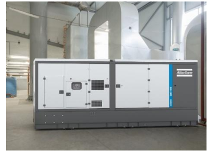
DIESEL POWER GENERATORS
